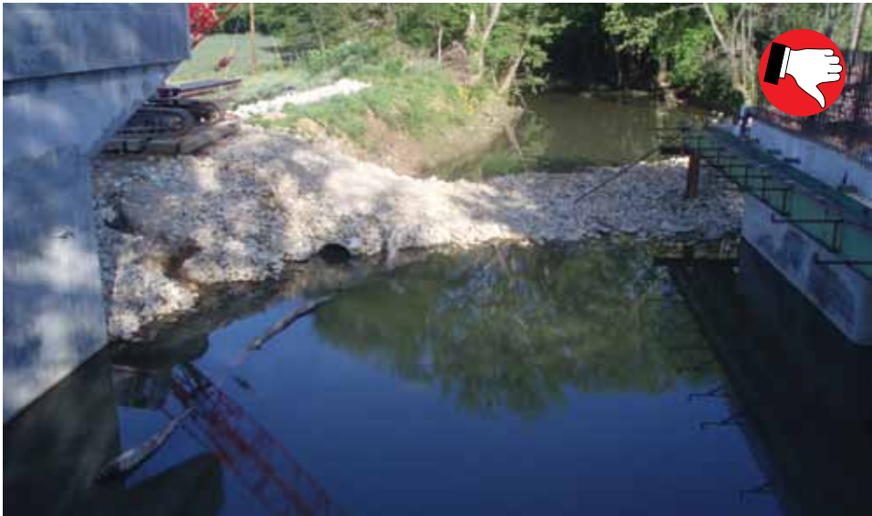
Pipes under temporary crossing are undersized causing creek to widen upstream.
