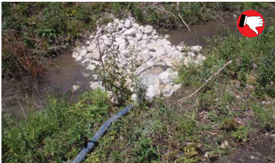
Stable outlet should not be placed in the stream channel. This is unpermitted fill and a violation of 401/404 permits.
