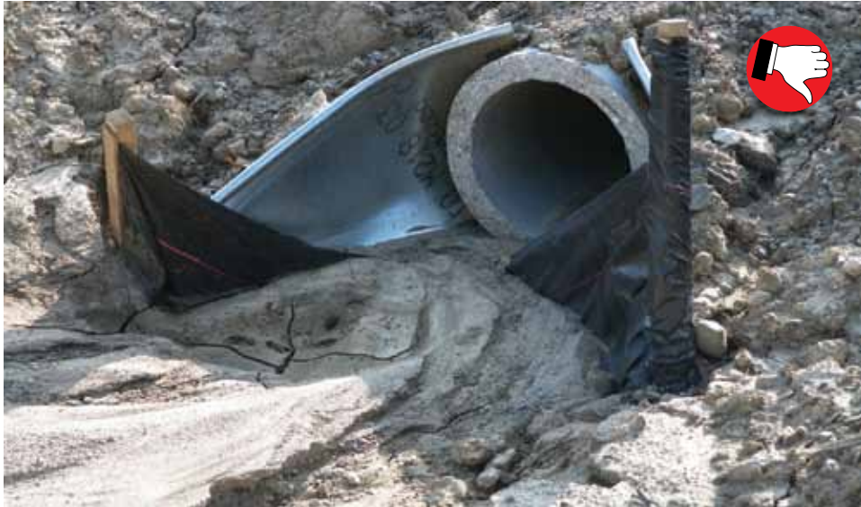
Silt fence should not be located in concentrated flow areas and is not appropriate as culvert inlet protection.
