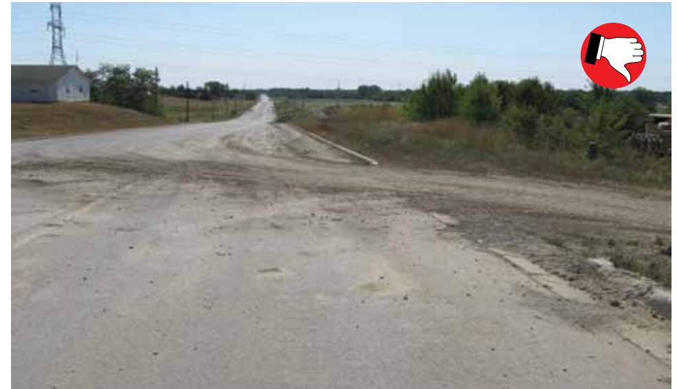
Insufficient #2 stone on construction entrance. Note tracking onto public roadway. Mud tracked onto paved roads is a common complaint from citizens.
