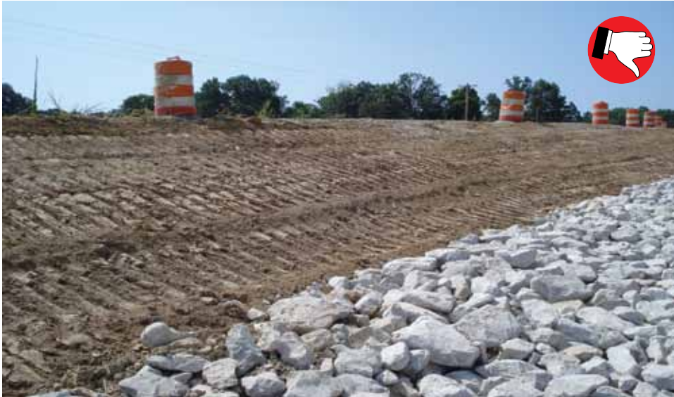
Vertical tracking will contribute to rill erosion.
