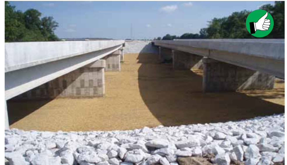
Picture showing adequate mulch cover per visual inspection. Mulch provides protection from erosion and retains moisture needed for seed germination and grass growth.
