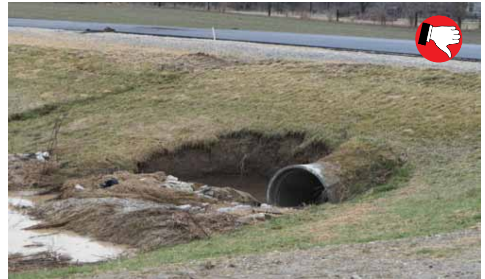
Culvert inlet protection not shaped correctly contributing to scour around inlet.
