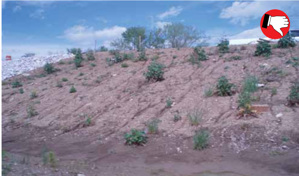
Weeds indicate slope has been unprotected. Temporary seed and mulch should have been applied within seven days of inactivity.
