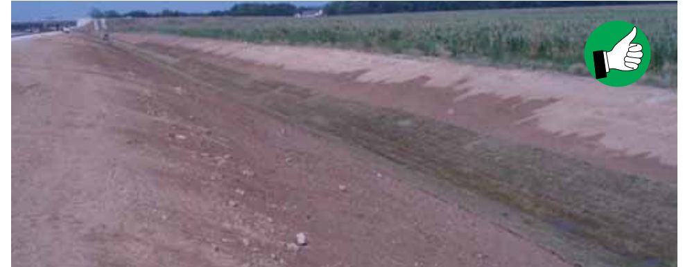
Sod installed in channel bottom with tight joints in the direction of water flow. Slopes should be stabilized to prevent sediment in the sod.
