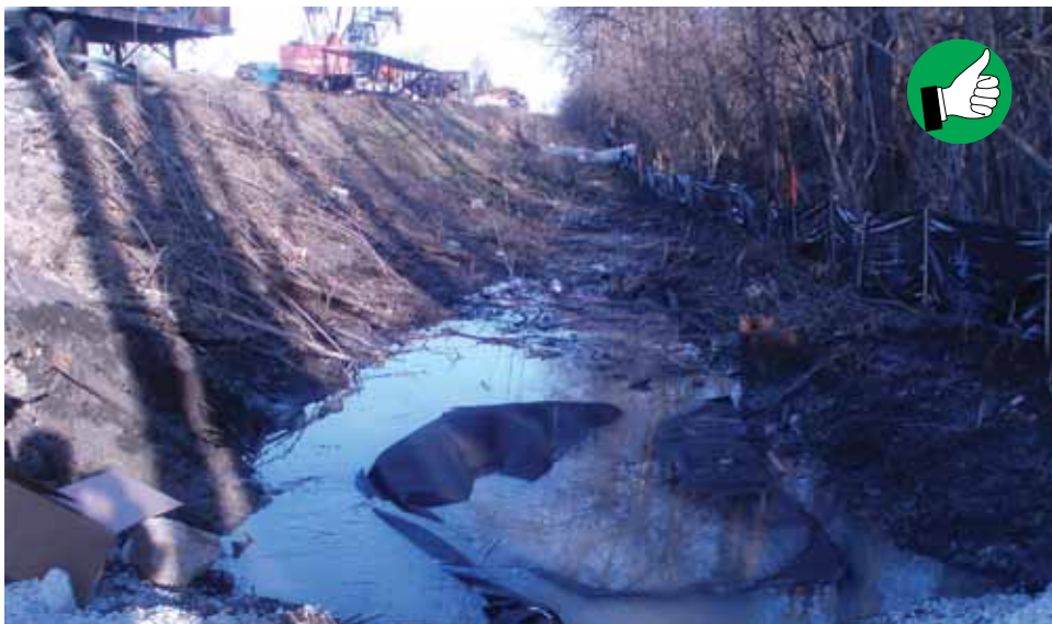
Filter bag and sediment trap used to filter sediment from dewatering operation.
