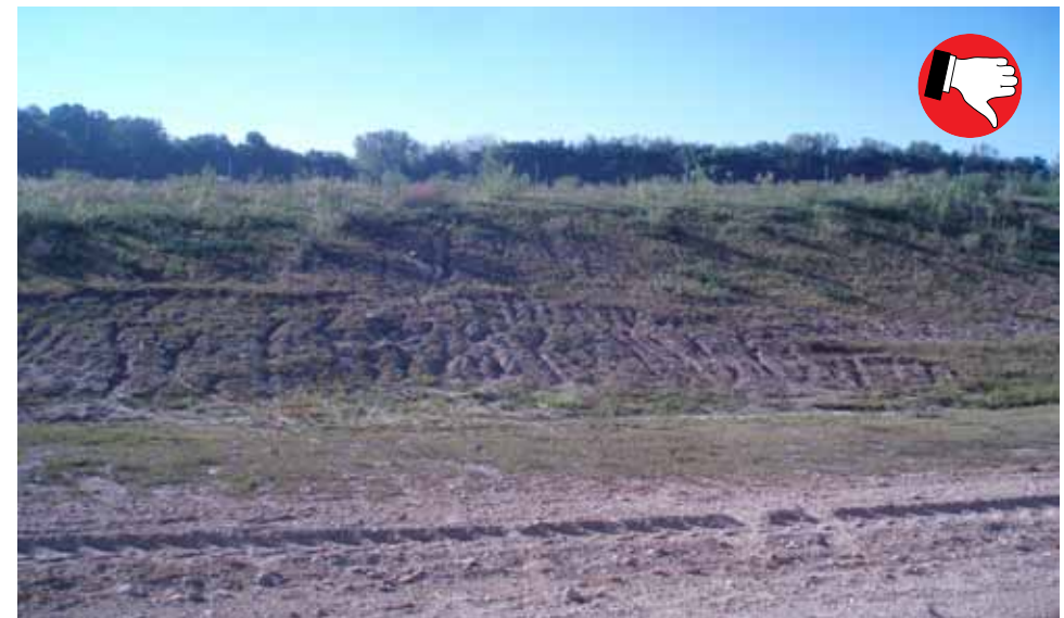
Vertical roughening of slopes makes erosion worse and creates a series of rills to quickly move water and sediment to the ditch bottom.
