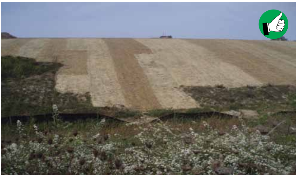
Erosion control blankets should be placed from toe to top of the slope on side slopes.
