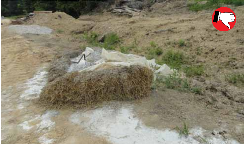
Concrete washout not contained.
