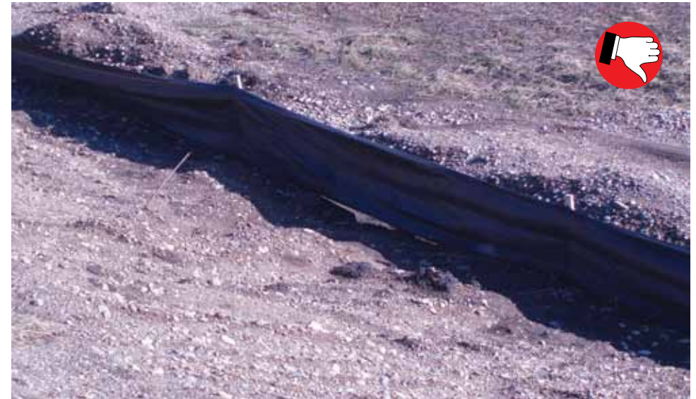
Silt fence not trenched in.
