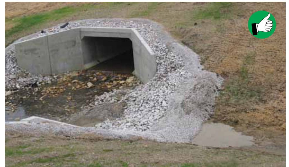
Sediment trap placed in an appropriate location close to stream with filter stone.
