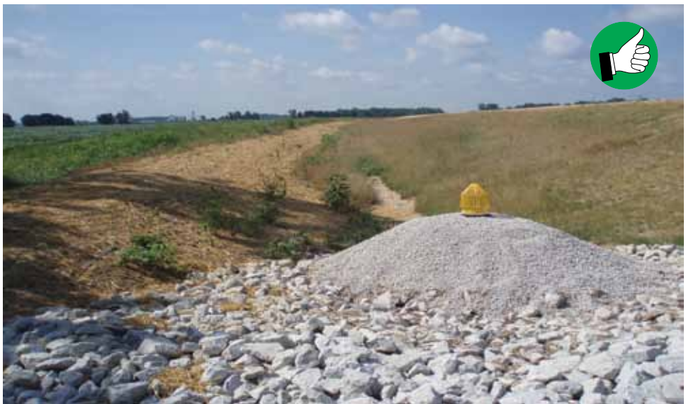
Sediment basin with stable slopes, stable outlet, filter stone and stand pipe. However, stand pipe installed too high as compared to surrounding land and outlet elevation.
