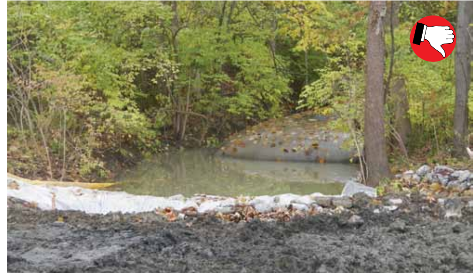
Filter bags should not be placed in waterways. Bags often break or become dislodged sending sediment downstream.
