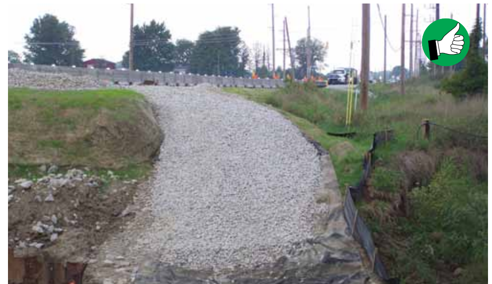
Construction entrance installed correctly, steep slope could not be avoided.
