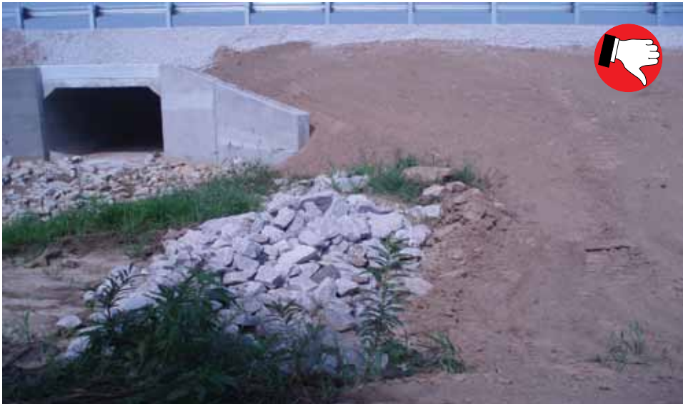
Sediment trap without filter stone allows sediment to travel through riprap and into waterway.
