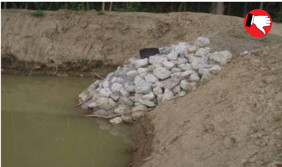
Sediment basin slopes are not stable and no filter stone is used on perforated stand pipe.
