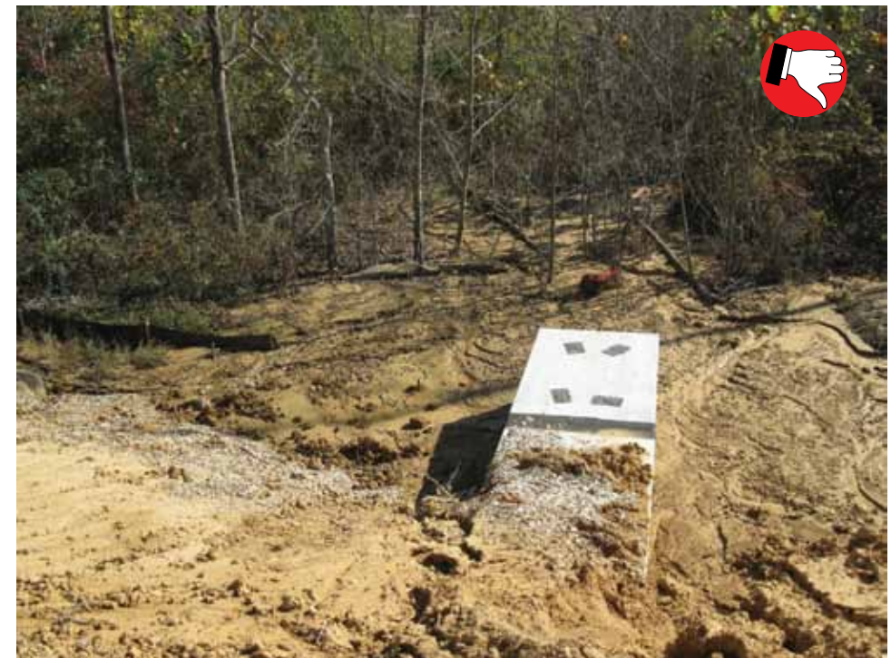
Sediment from construction site filling in a stream. This is a violation of many environmental permits.
