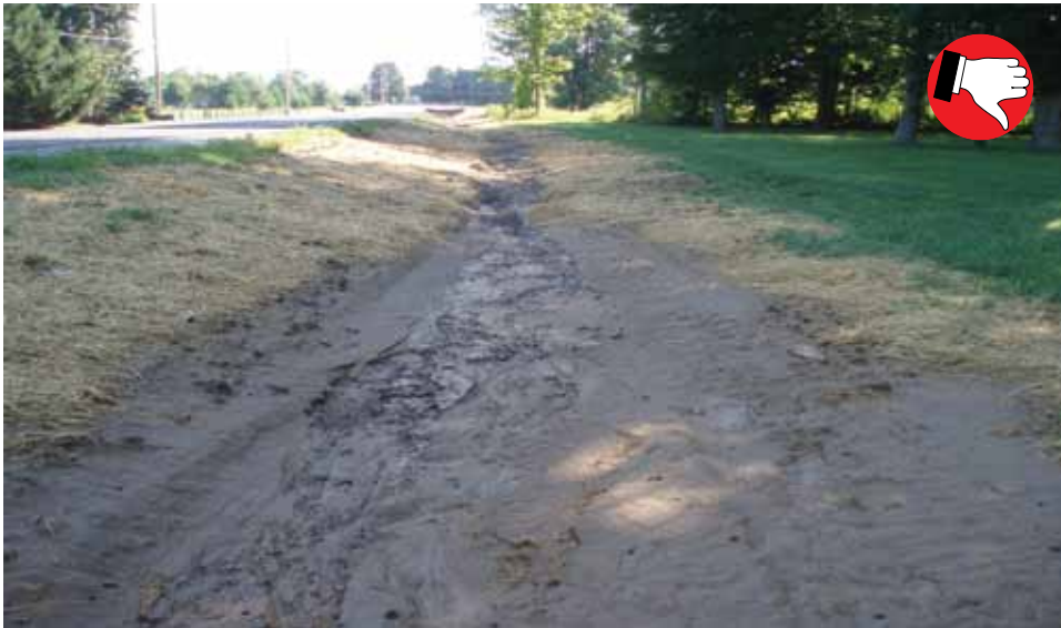
Ditches without blankets will wash the mulch away, disabling grass from growing and leading to erosion.
