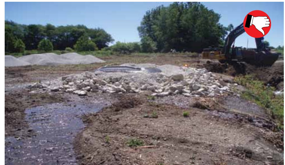
Pump around water does not need to be filtered. This filter bag and secondary containment is intended for the dewatering operations.
