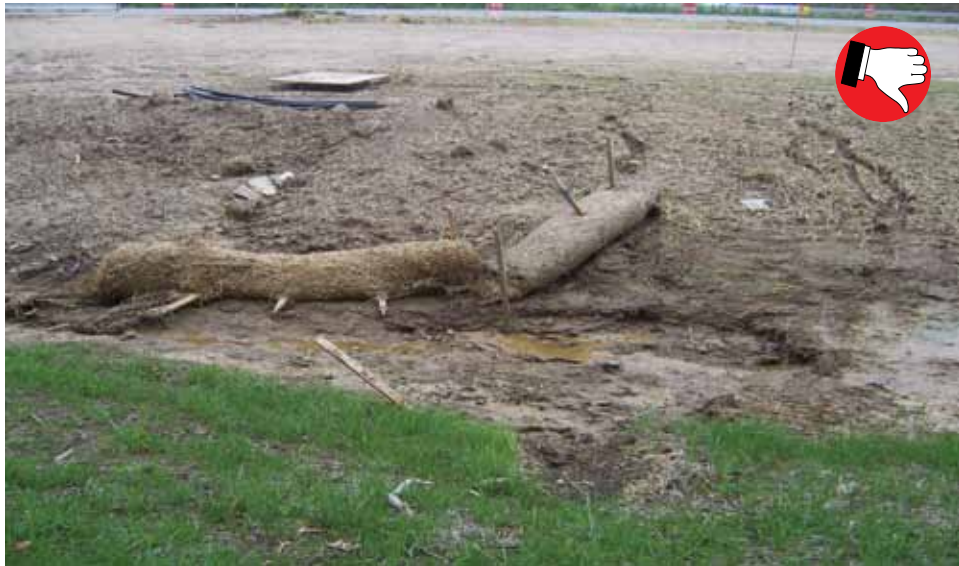
Filter sock used as traversable check dam in the clear zone (good) but installed where water velocity is very high (bad). No geotextile was used and only one filter sock was used (verses three in a pyramid).
