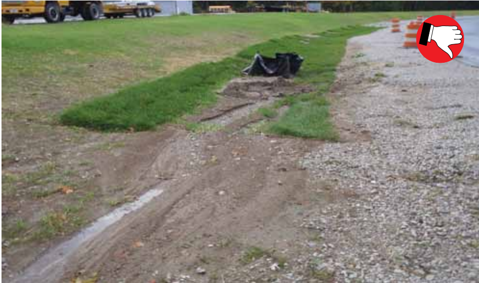
Area upstream of sodded ditch is not stable and causing sedimentation on permanent sod.
