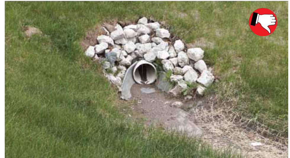
Permanent inlet protection without Geotextile fabric and haphazard placement.
