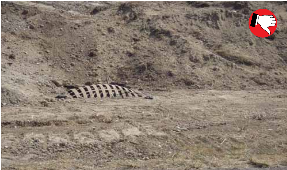
Geotextile placed under inlet is not an acceptable inlet protection measure. Geotextile will clog causing standing water, making measure impossible to maintain without getting muddy water into storm system. Ponding water could cause traffic hazards or muddy construction conditions.
