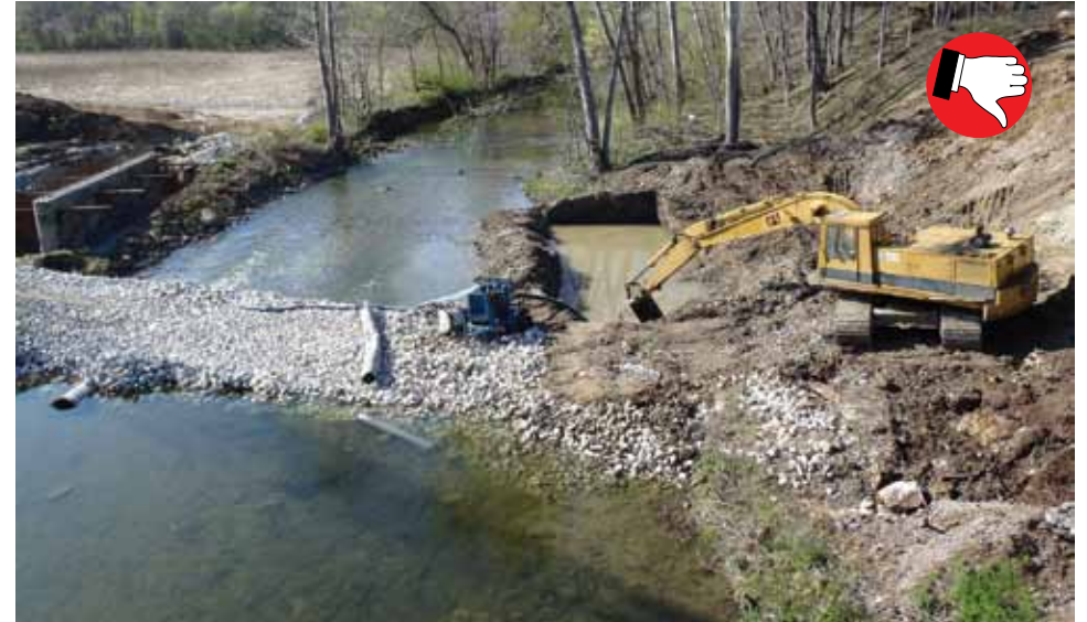
Bare earth is highly erodible and not a suitable barrier to be used for cofferdams. Water infiltration is evident.
