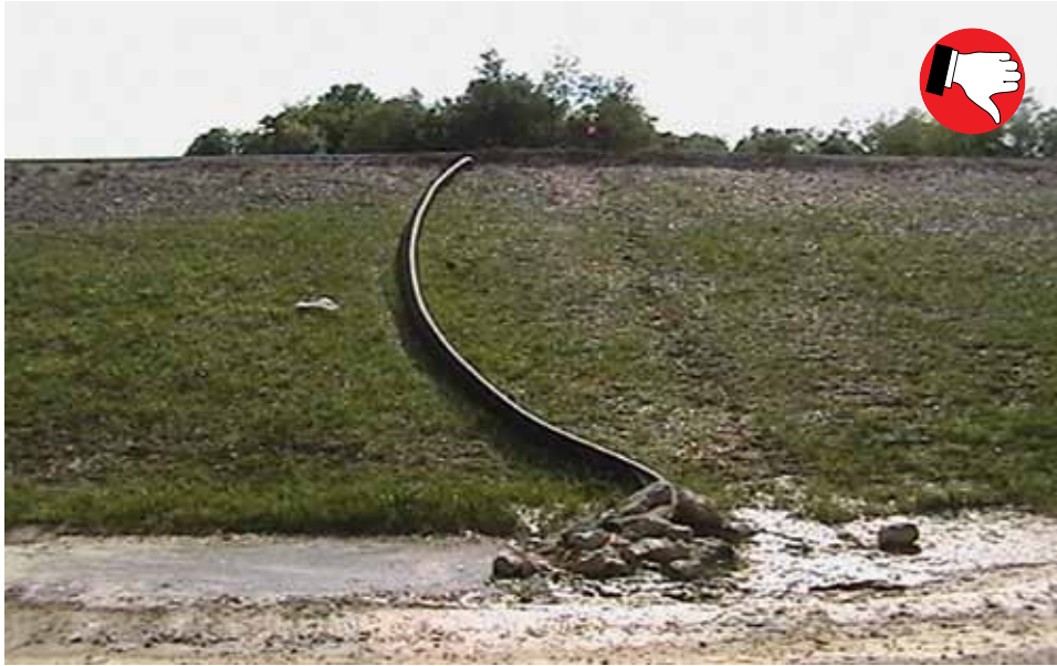
Slope drain is functioning; however it is not properly anchored.
