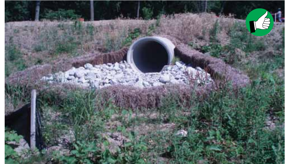
Although not an INDOT standard, straw bales and riprap functioning well for culvert inlet protection.
