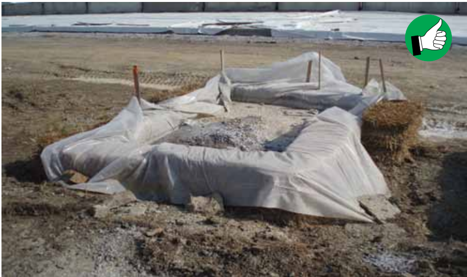
Concrete washout that is properly contained, close to capacity and appropriately located along access road.
