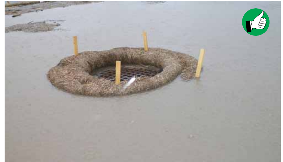
Filter sock inlet protection staked correctly.
