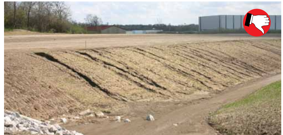
Slope erosion caused by lack of slope drain installation.
