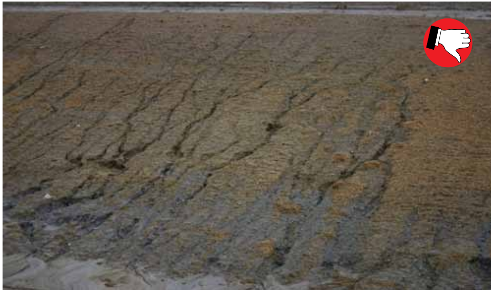
Temporary mulch applied too thin contributing to erosion. Application rate should be 2.5 tons per acre.
