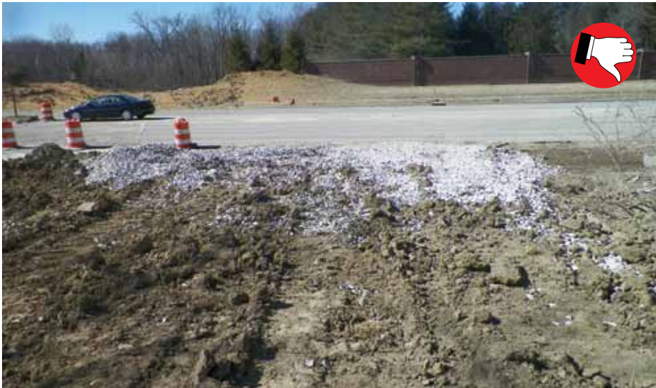
Construction entrance not the minimum 50' long.
