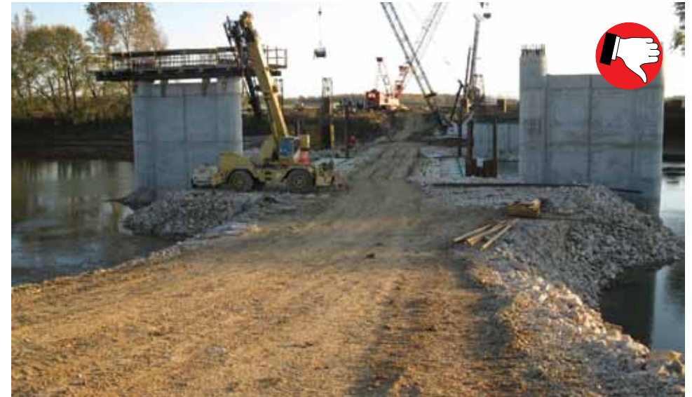
#2 stone on temporary crossing needs to be redressed to reduce sediment entering creek during rain events.
