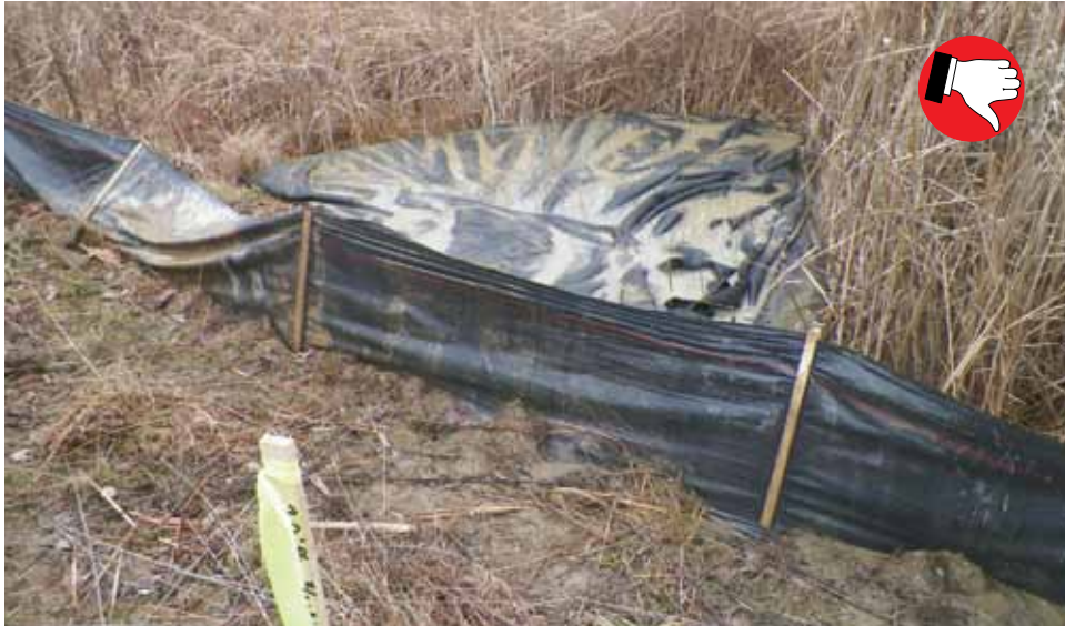
Filter bag has been placed outside construction limits and in a jurisdictional wetland. This would be considered a permit violation and cause for work stoppage and possible fines.
