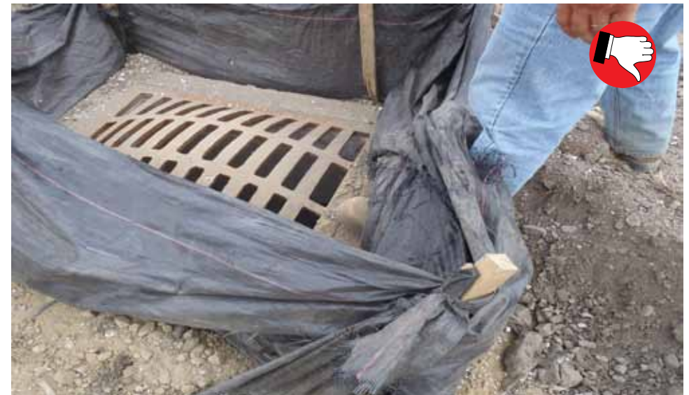
No cross bracing used on inlet protection. Silt fence not trenched properly.
