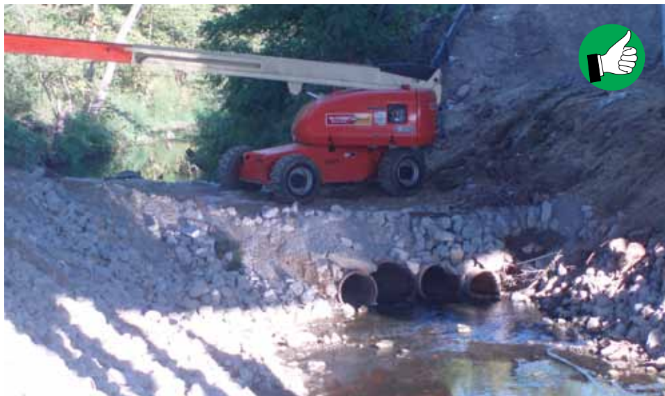
Temporary crossing with adequate pipe capacity. These temporary impacts must be permitted, usually by the contractor, prior to installation and should be removed as soon as practical.
