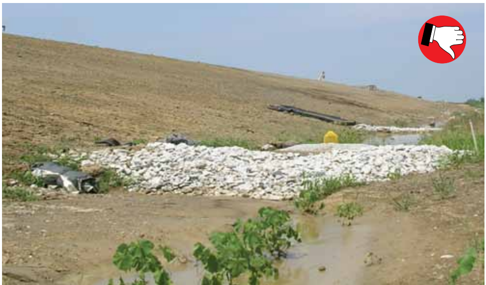
Sediment basin overflow pipe is installed too high. Pipe opening should be at least 2' below the stable overflow weir. Basin not sized to handle 5+ acre watershed.
