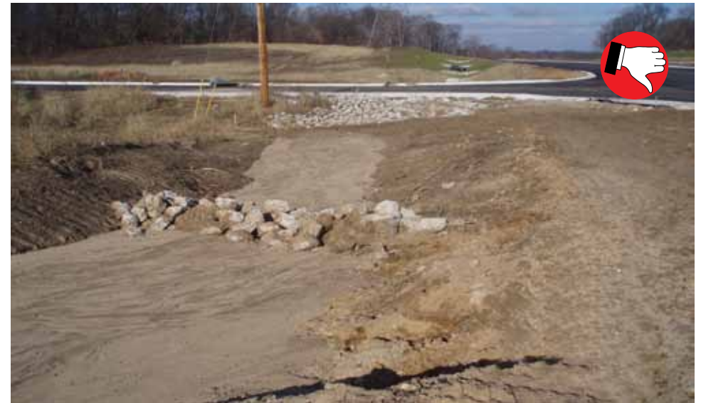
Rock check dam not built to specification. Not shaped correctly, no filter stone, no Geotextile.
