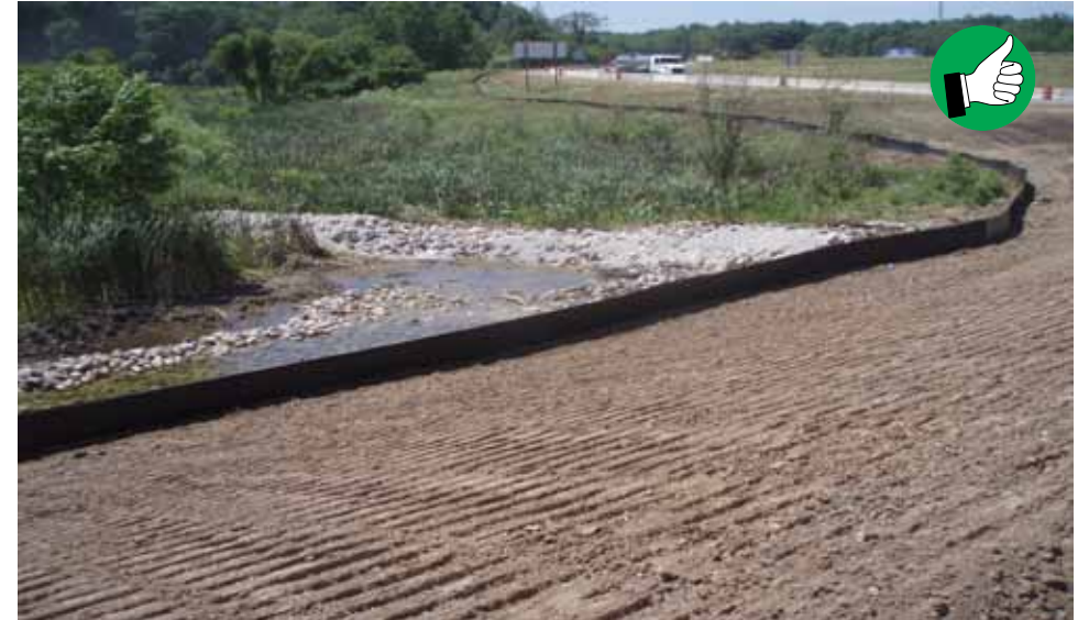
Horizontal tracking of slopes create small ridges and valleys to trap seed and mulch and help stabilize a slope.
