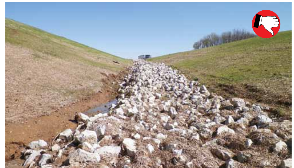
Riprap is not extended far enough up the slope and not shaped correctly, causing scour.
