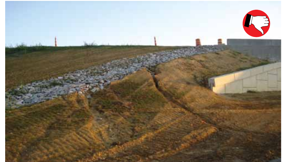
Rock chute installed without proper swale depression causing erosion rills.
