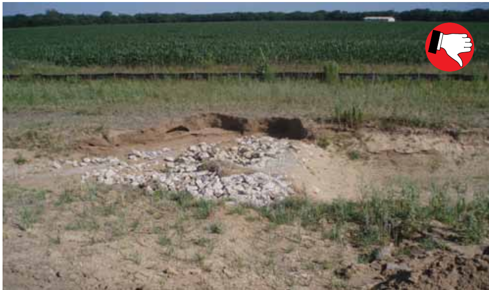
Check dam not shaped correctly causing water to bypass dam and erode slopes.
