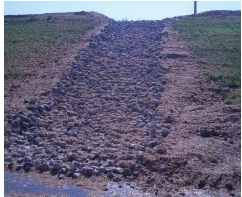
Off-site water managed with a diversion interceptor and rock chute.
