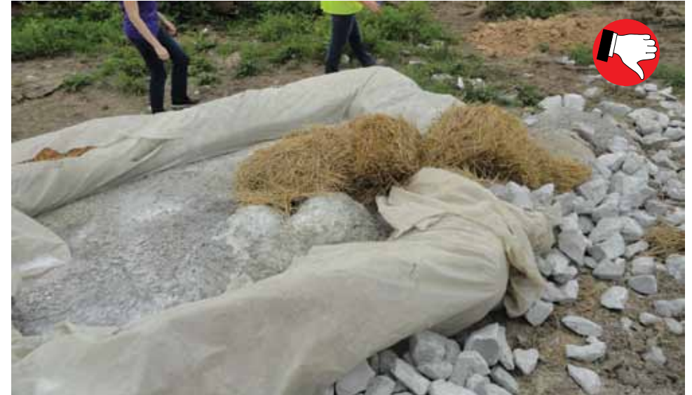
Concrete washout should have one continuous sheet of plastic. Overlapping layers allows chemicals access to the soil below.
