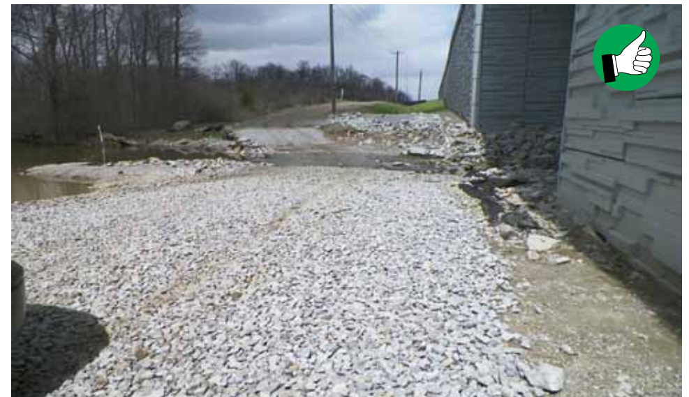
Construction entrance with geotextile and #2 stone constructed from road to temporary crossing to stabilize slope and reduce sediment tracking to the waterway.
