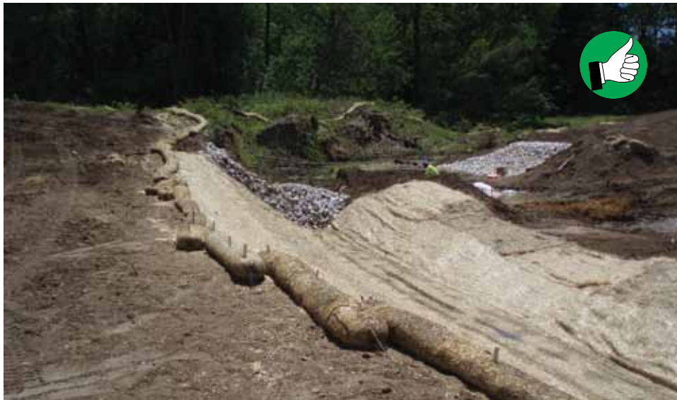
Stable diversion interceptor around a box culver installation. Diverted stream water should flow freely. Riprap should not be placed in channel.
