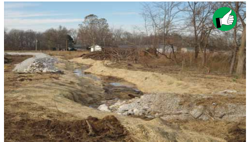
Blankets can be used as temporary or permanent erosion control around hot spots such as creek banks.
