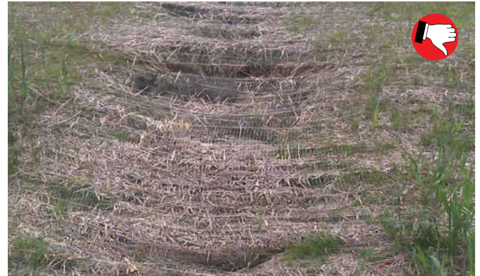
Erosion control blankets will not work if proper soil and soil grading is not completed first. Blankets not installed parallel to direction of water flow.
