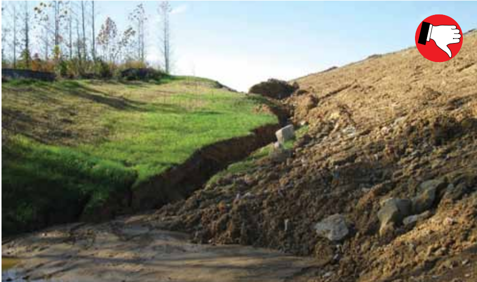
Permanent riprap should be installed in steep ditches to prevent gully erosion.
