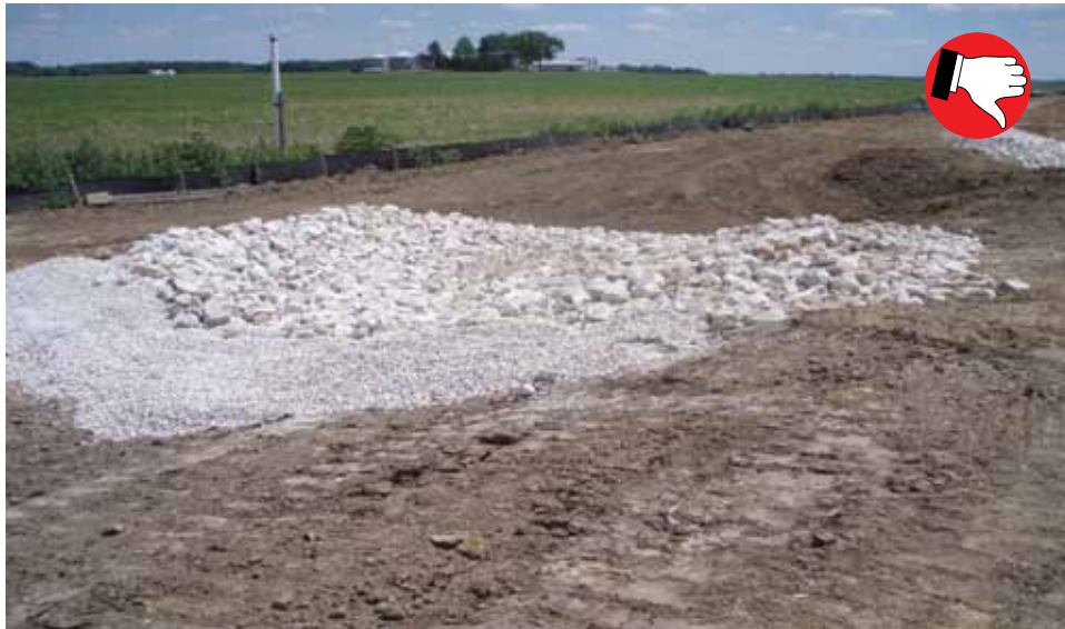
Check dam is much bigger than necessary.
