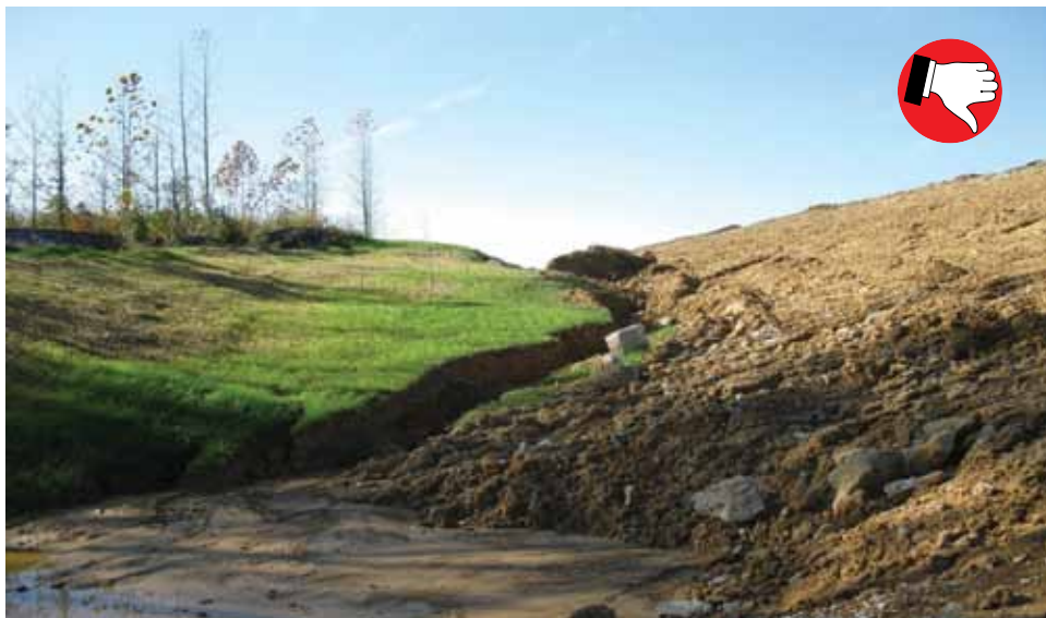
Rock chutes should have been used to stabilize slope. Erosion is causing large rills to form and sediment transportation is evident.
