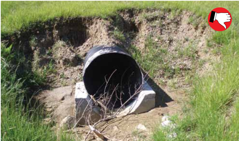
The lack of permanent protection has caused scouring around pipe inlet.
